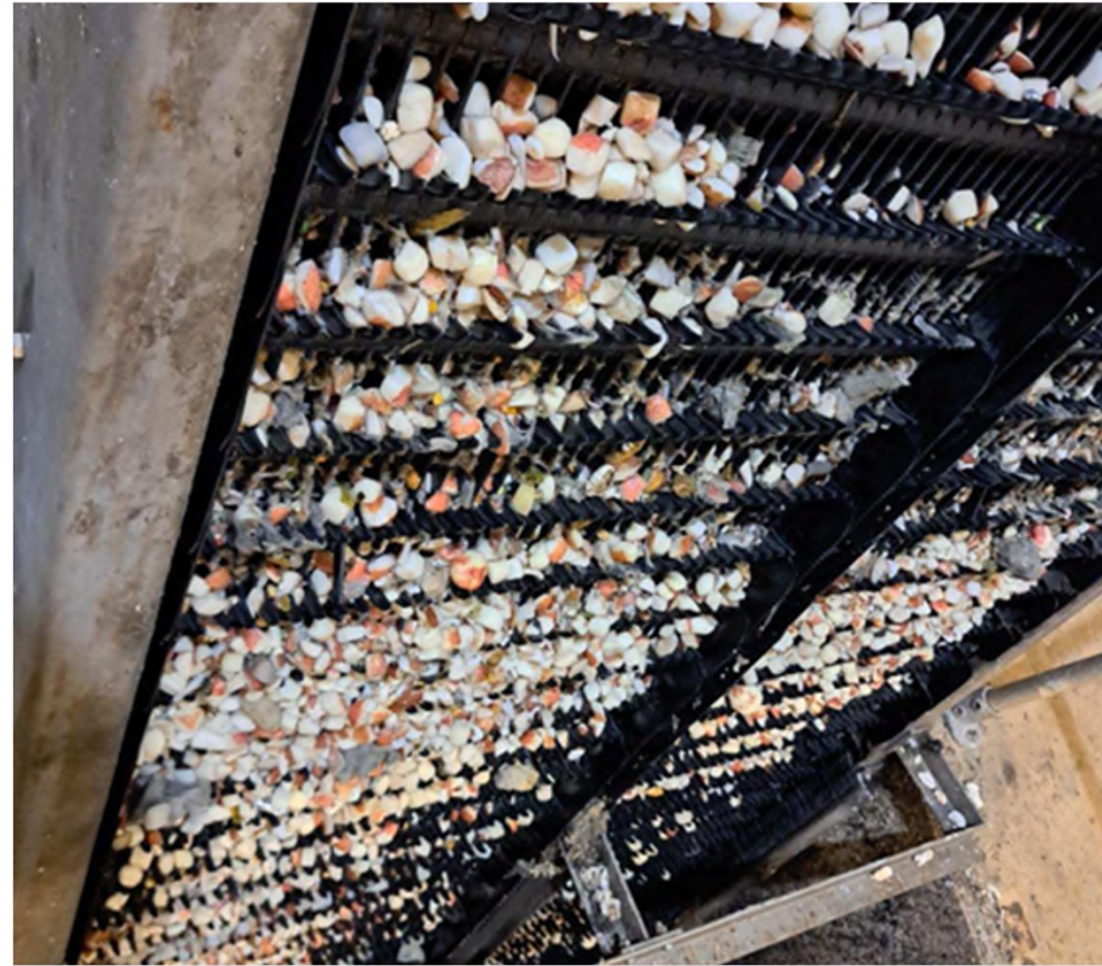
Bar Screen - Slug Discharge
